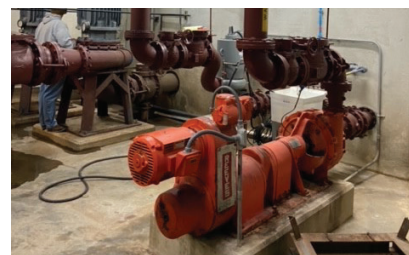
Before installation of new pump
